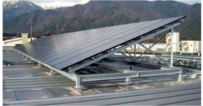
DDS Komagane Plant (20kW, FY2008 operation start)
