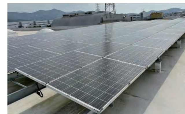
Topura Hadano Plant (20kW, Start from FY2012)
